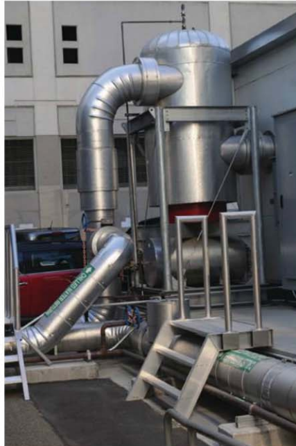
Outside chilled water system
